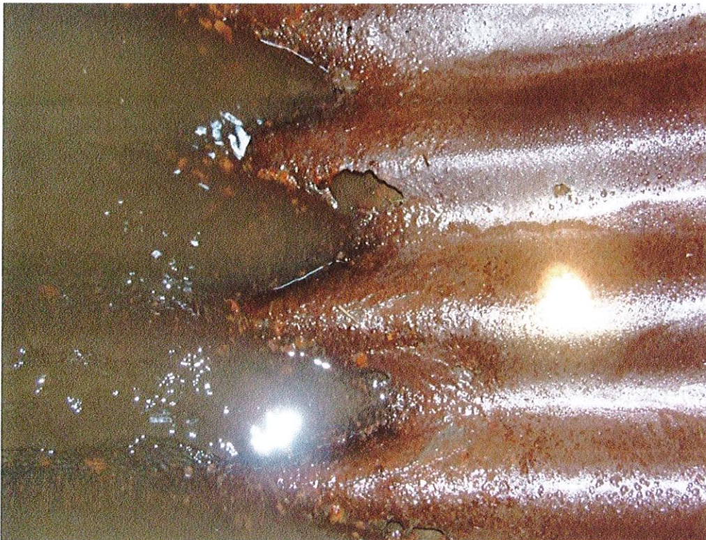
Photo 20. Typical perforation at culvert bottom in section 4
