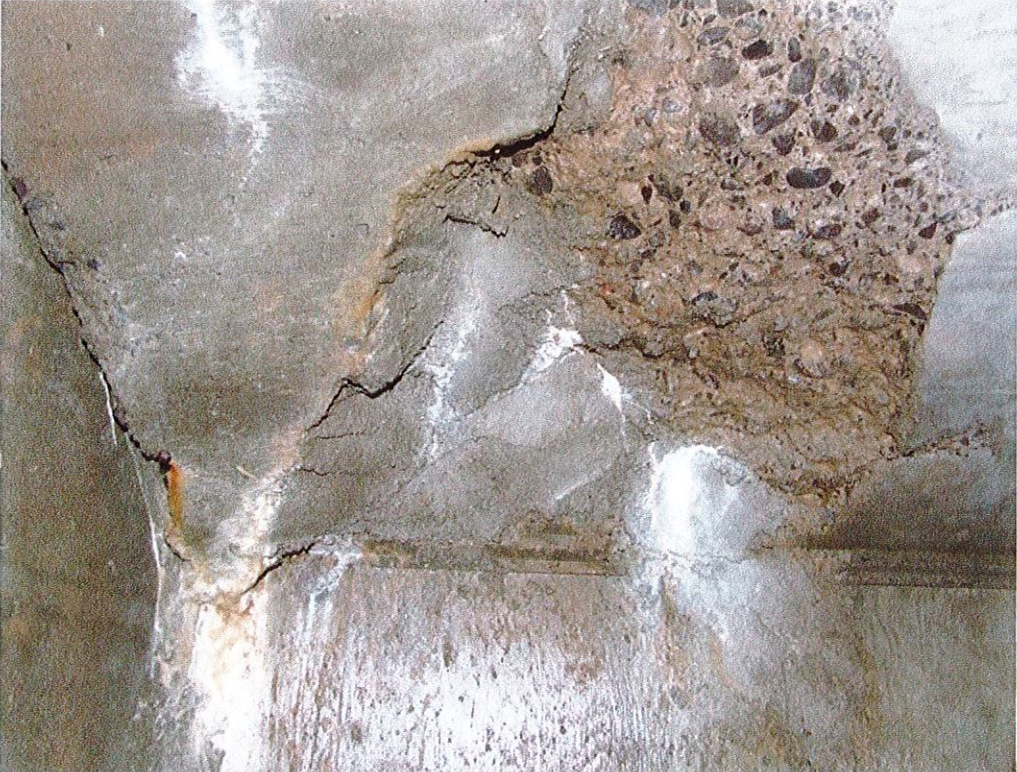
Photo 12. Scaling/spalling at the upper southwest corner
