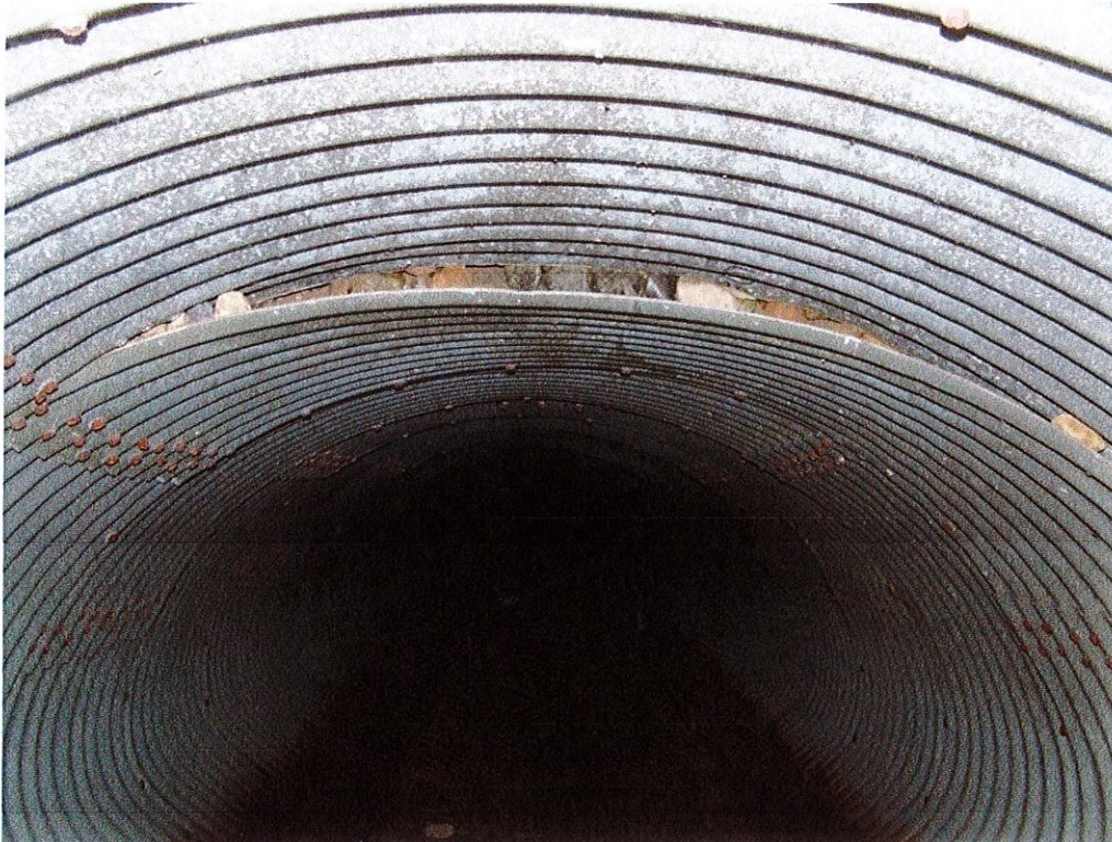
Photo 5. Deflection/opened plate joint
