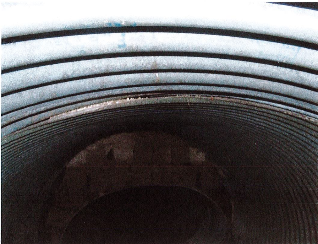
Photo 16. Minor erosion through plate joint
