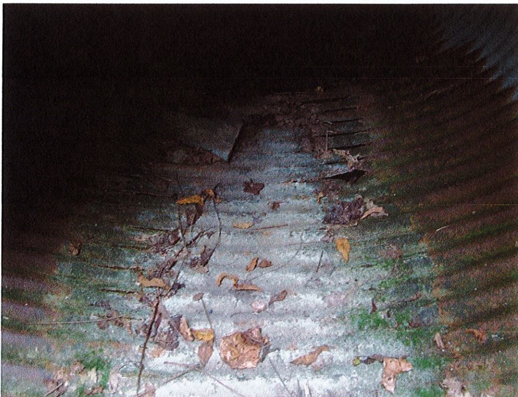
Photo 4. Severe corrosion, perforation, and heaving at inlet bottom
