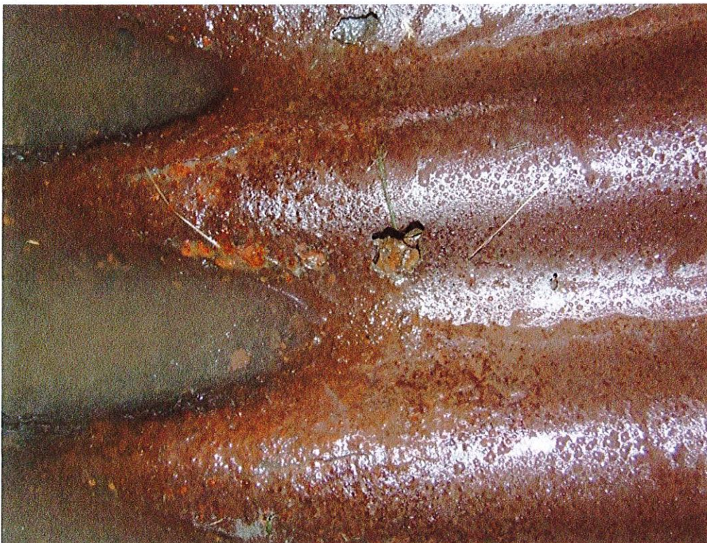
Photo 18. Typical perforation at culvert bottom in section 4
