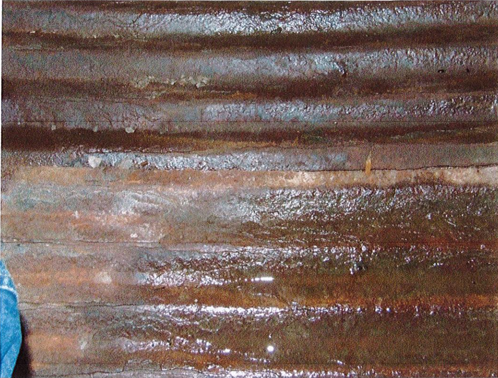
Photo 7. Close-up view of the corrosion in photo 6
