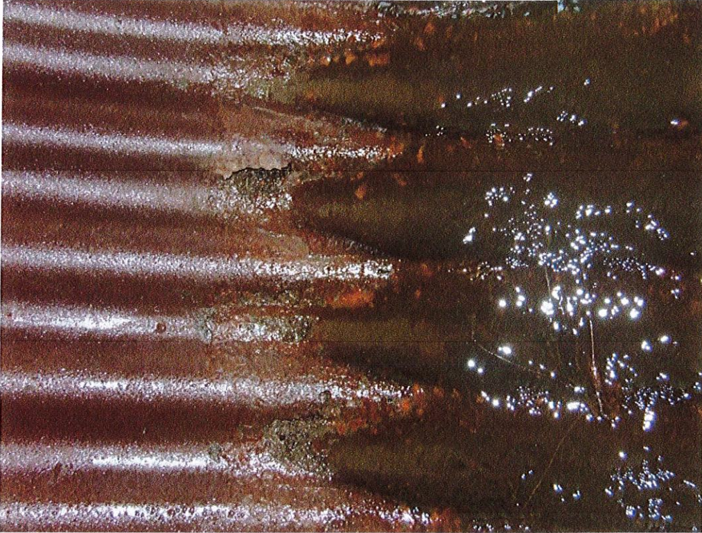
Photo 19. Typical perforation at culvert bottom in section 4
