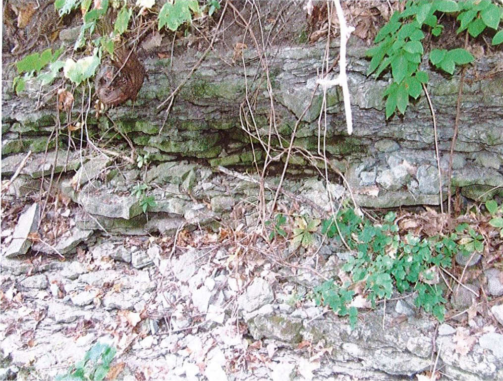
Photo 3. Erosion of creek embankment
